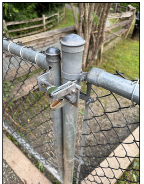
Broken gate latch
